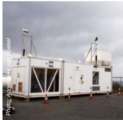
The StatoilHydro hydrogen plant at Utsira.
