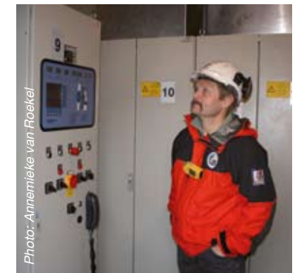
A worker of StatoilHydro checks the meters inside the Utsira hydrogen plant.
